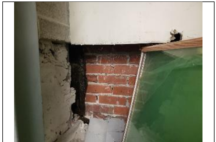
12. Non-asbestos tar paper present in Room 123.
