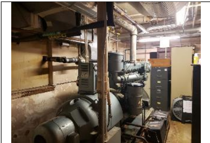
5. Room 125, lead paint present.
