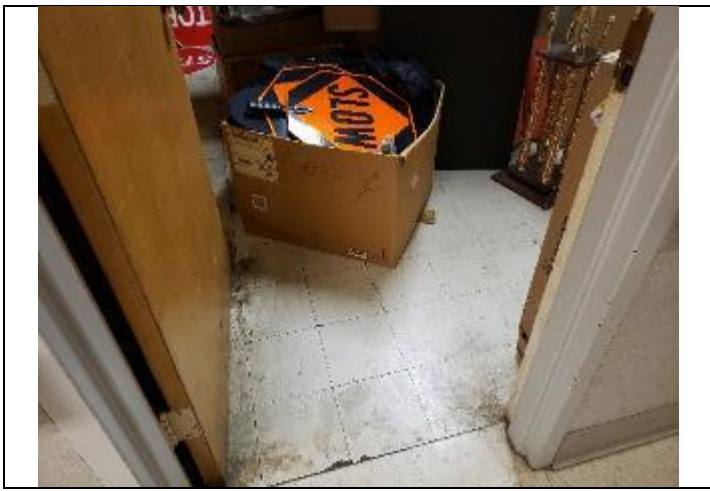
1. Room 137, ACBM white 9” floor tile and mastic present.
