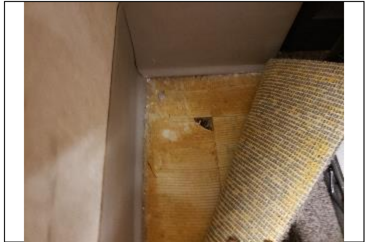
4. ACBM white 9” floor tile and mastic present under the carpet in Room 135.
