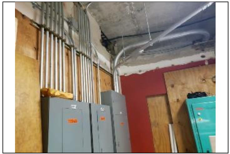
2. Room 137, electrical components present.
